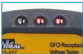
Red Lights Indicate Incorrect Wiring
