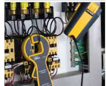
Inductive clamp allows you to induce a tracer signal on to the cable without affecting the low voltage signals on the circuit.
